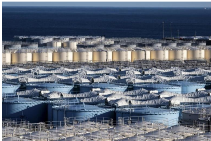
Figure 1: Storage tanks for contaminated water at Fukushima Daiichi nuclear power plant, January 20, 2023. © Philip Fong, AFP
